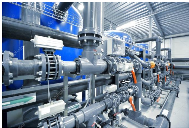
Figure 1. Water treatment machines use a variety of industrial minerals to make water safe for consumption.
